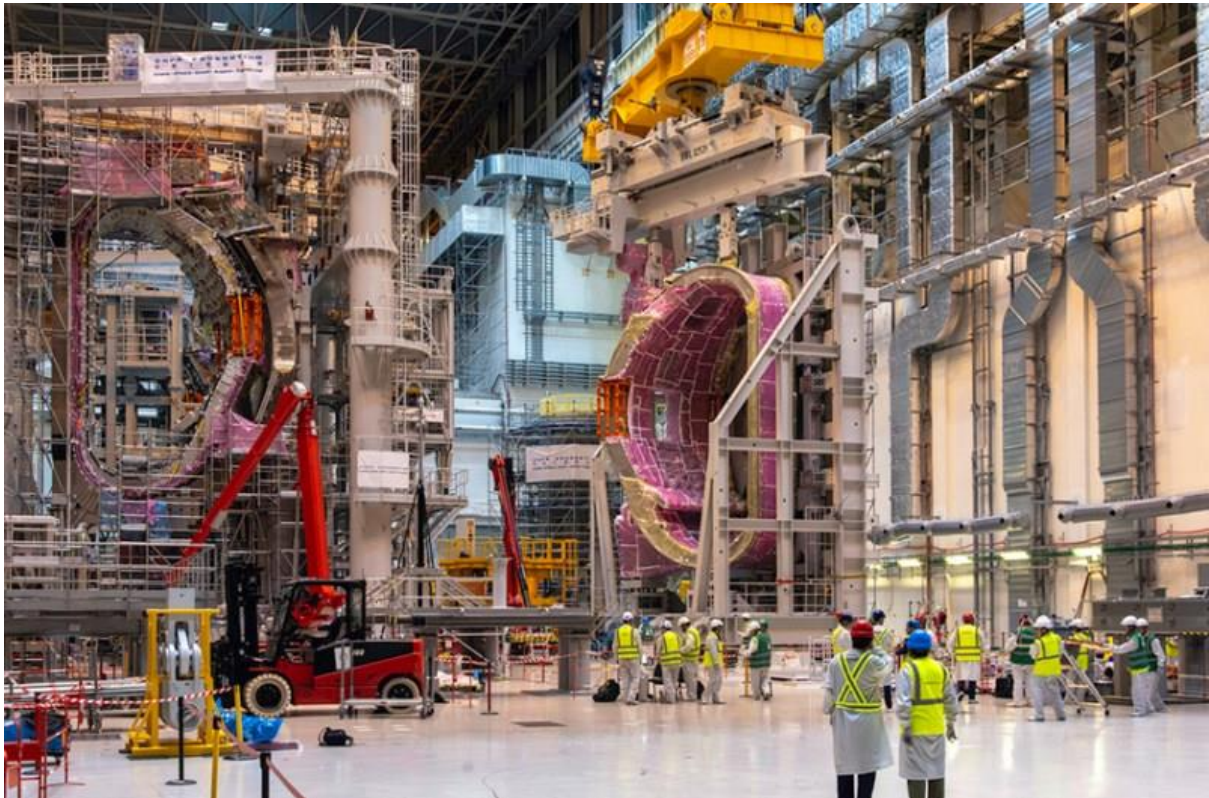
A current view of the ITER Assembly Hall 3 sectors in the tokamak pit, where vacuum vessel sectors and large magnets can be seen in stages of tokamak pre-assembly
